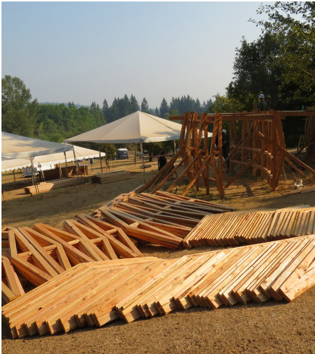
Figure 2: Wooden trusses, constructed by students, being used in their initial iteration as part of a temporary, outdoor performance venue.
