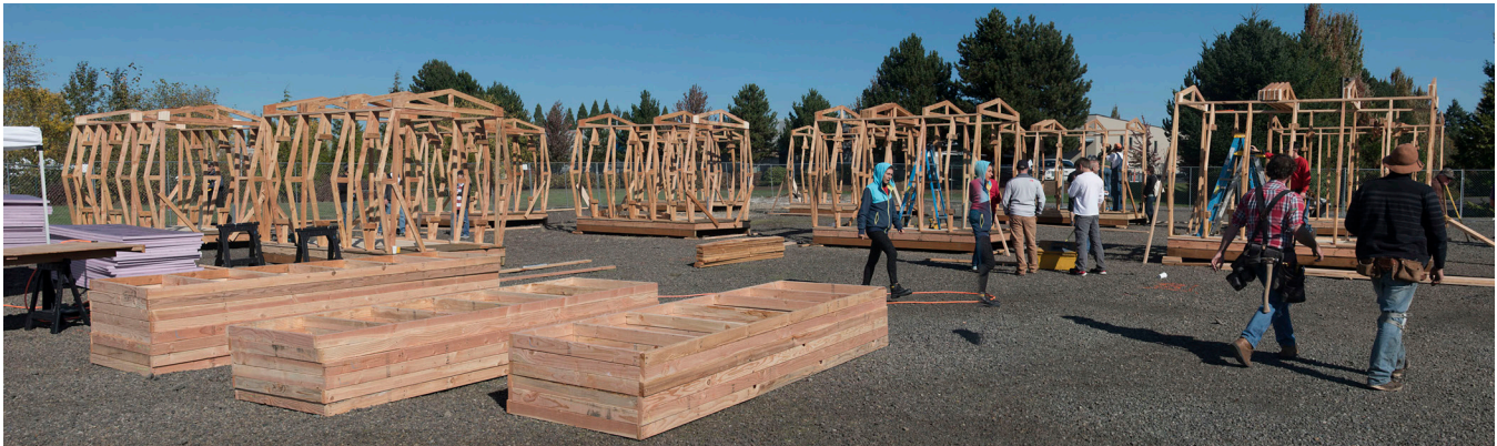
Figure 1: Wooden trusses being utilized in their final iteration as the structural frame for new homeless sleeping PODs.
